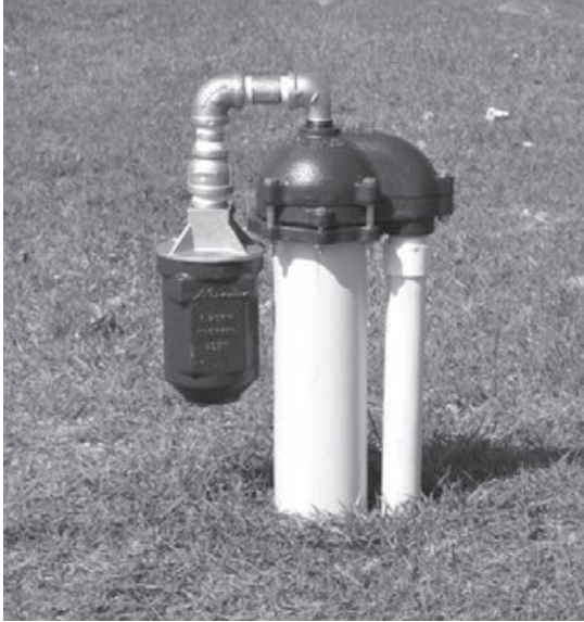
Drilled well with flood-protected cap
