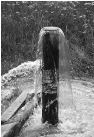
Flowing well that is not controlled.
