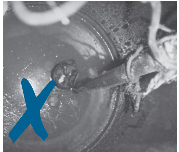
Surface water in well pit.
